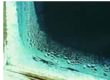
Window condensation can fuel mold growth.
